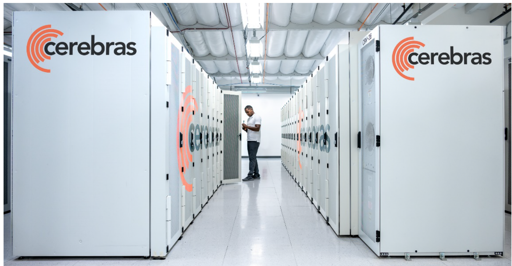
Figure 3. Cerebras Cluster installed in a datacenter.
